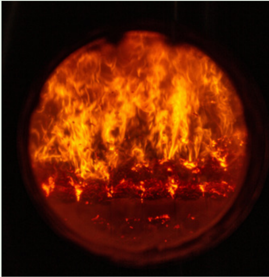
Biomass: Wood chips boiler
